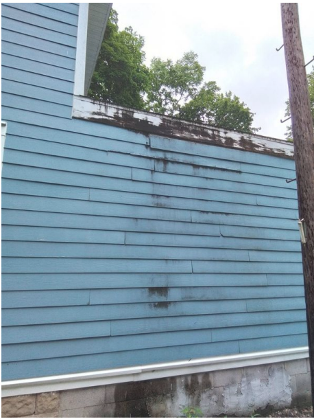
1st Floor right side. No overhang allows roof runoff to run down side of house.
