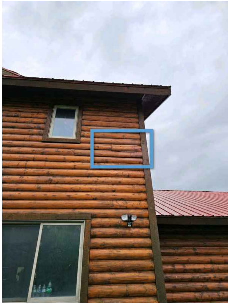
Repaired as of 5/29
