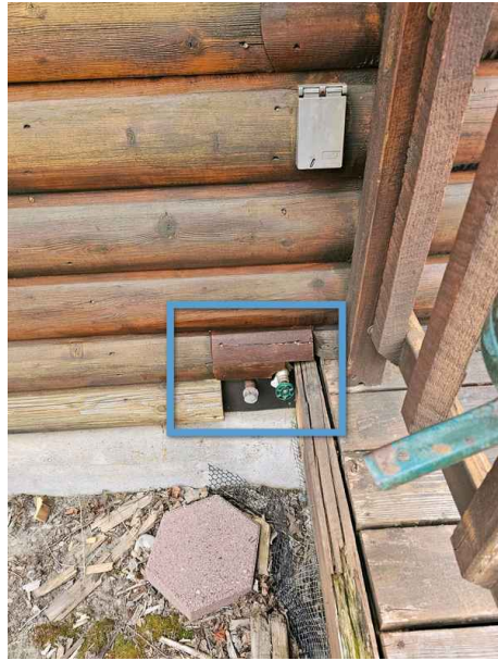
Repaired as of 5/29
